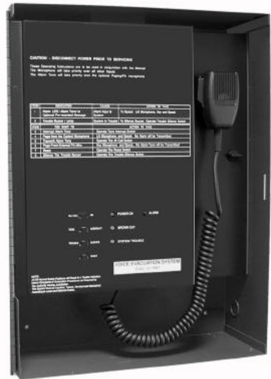
Shown with Key locked Door Removed
