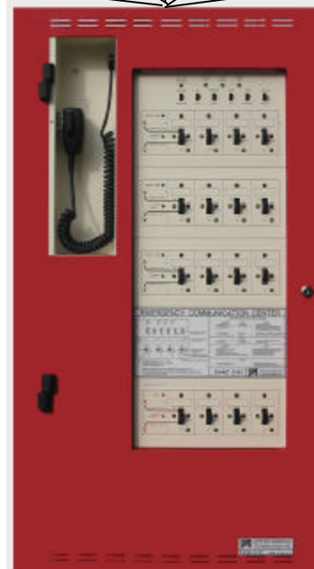
MASS EVAC MAIN CONTROL
